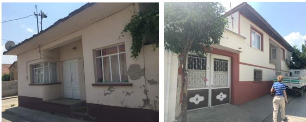
Figure 4.19 Republican architecture 1story and 1 story with basement (Right one Appendix-G Left one Appendix-E) (Auror 2013-2017)
